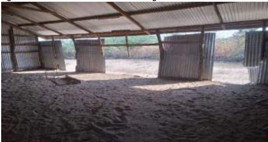
Figure 22 b. An ECDE Classroom with damaged iron sheets walls
