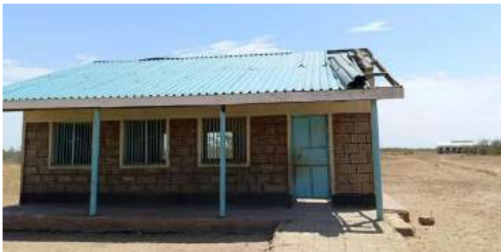
Figure 2.4 b A classroom roof that had been completely blown away by the strong winds.
