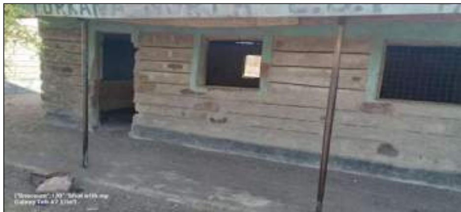
Figure 27. Dilapidated Classrooms with Doors, windows
