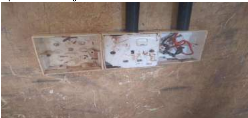
Exposed electrical fittings in an ECDE centre
