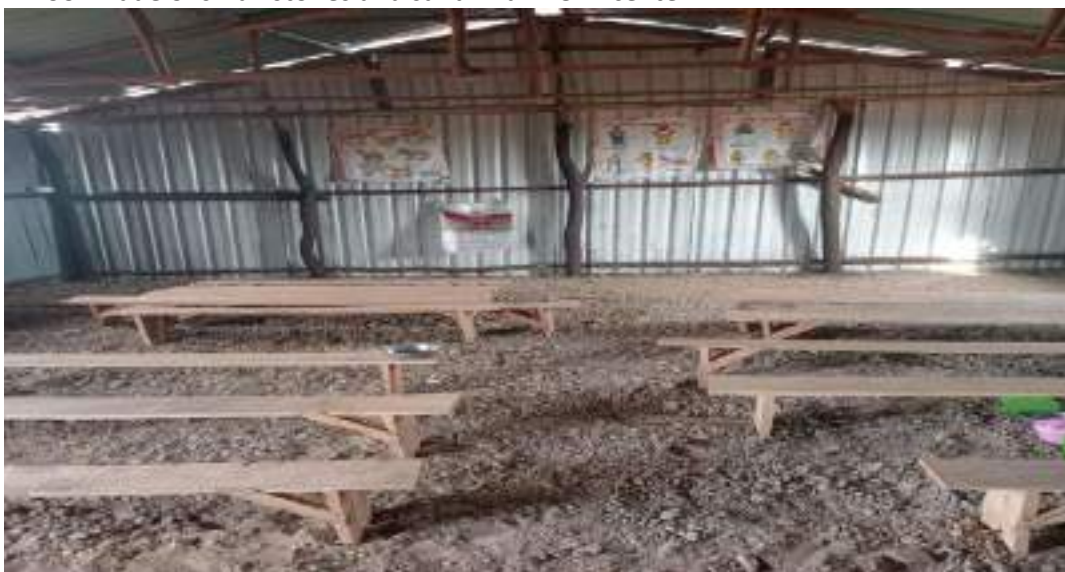
A floor made of small stones and sand in an ECDE center
