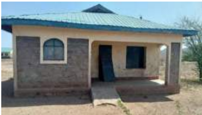
Figure 31. Poorly Constructed Ramp for Classroom Access
